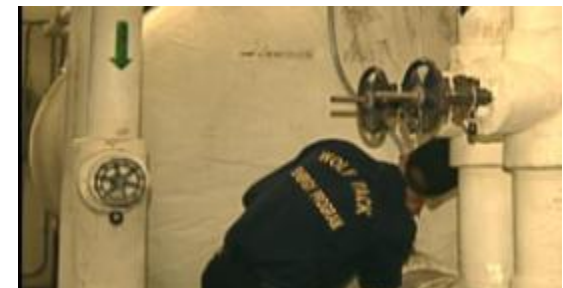
Kunsan Contract Resource Efficiency Manager -- ID'd & fixed excessive temperature in gym's hot water system, saved $7K per year. No-cost-low-cost.
