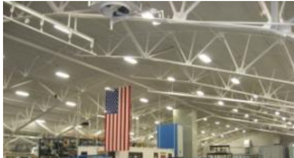
Elmendorf B8326 Air Ground Equipment Maintenance -- T5 High Output Lighting, PACAF SRM
